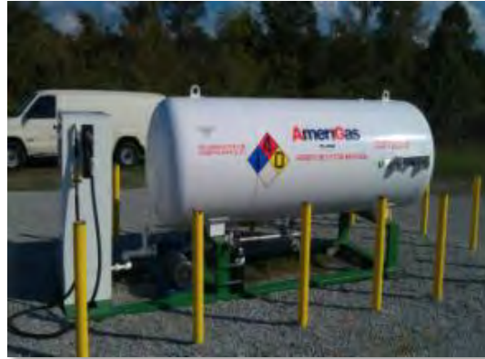
AmeriGas Propane Tank
