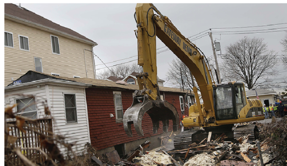
A Staten Island home damaged by Sandy is demolished. | AP Photo/Seth Wenig
